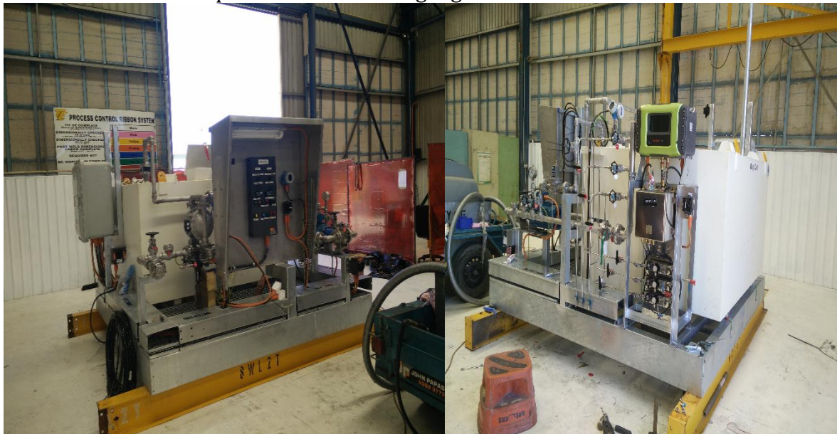
Figure 1: Diesel Additive Skid
