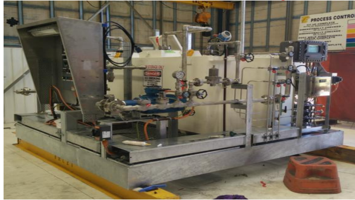
Figure 12: Work Setup of diesel additive skid
