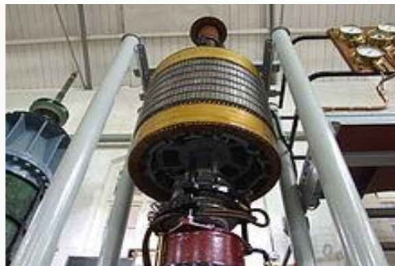
Figure 6: Rotor of a large water pump. The slip rings can be seen below the rotor drum.
