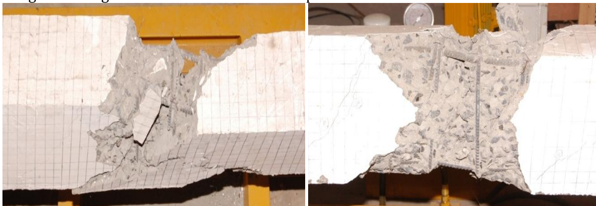
Figure 6: Failure of conventional steel reinforced beams due to yielding of longitudinal and transverse steel ( Bp_1m_1F_e )
